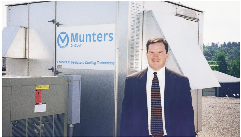
Paul Joslyn, energy manager for P&C Foods, stands next to Munters' desiccant SuperAire system which was retrofitted to their existing unit.
