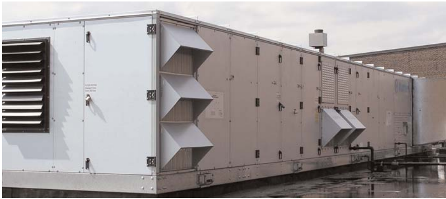
The AM20-1300G at Centennial is the first Munters' unit for a large scale pool application to be sold in Canada.
